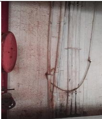
Old Conduit and Hanging wire
